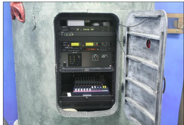
Similar interfaces for technical systems in each room makes training volunteers easy.
